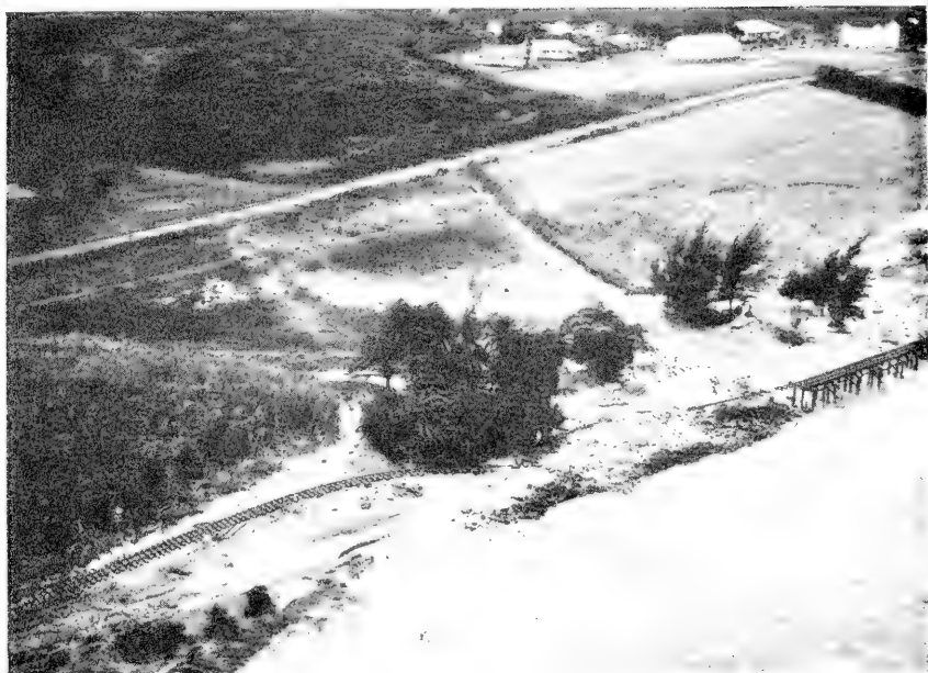
1. RAILROAD TRACK SWEEPED INLAND FROM ITS BED AT WAIALEE, OAHU Photograph by U. S. Navy.
